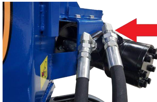
Both hoses connected at the hydraulic motor
