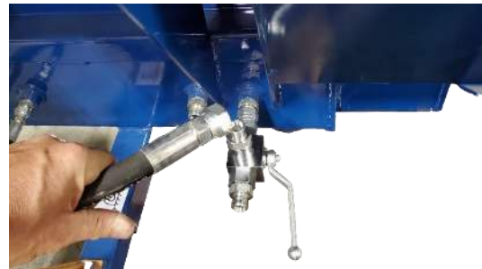
Valve installed and original hose connected to the middle fitting
